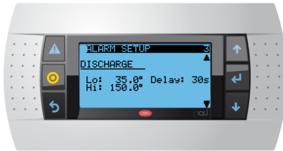
Figure 19 Discharge alarm setpoints
